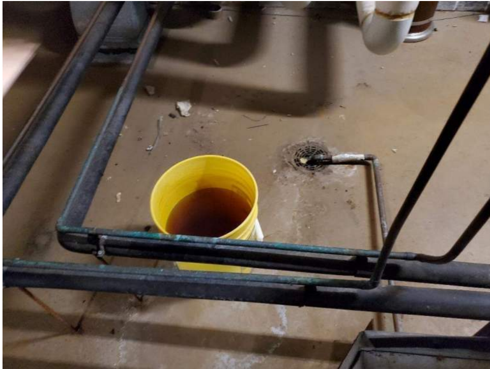
Photograph 21 – Mezzanine surface drain and 5-gallon bucket 2/3 full of leaking water.
