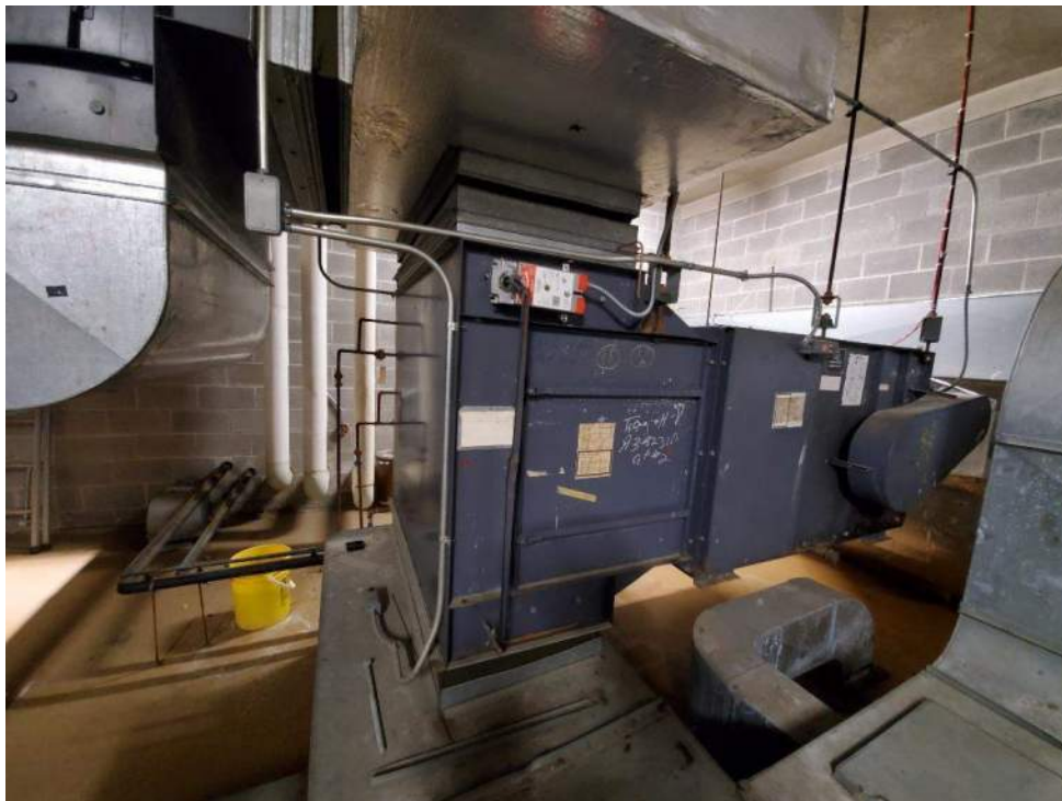
Photograph 20 – Mezzanine air handling unit.
