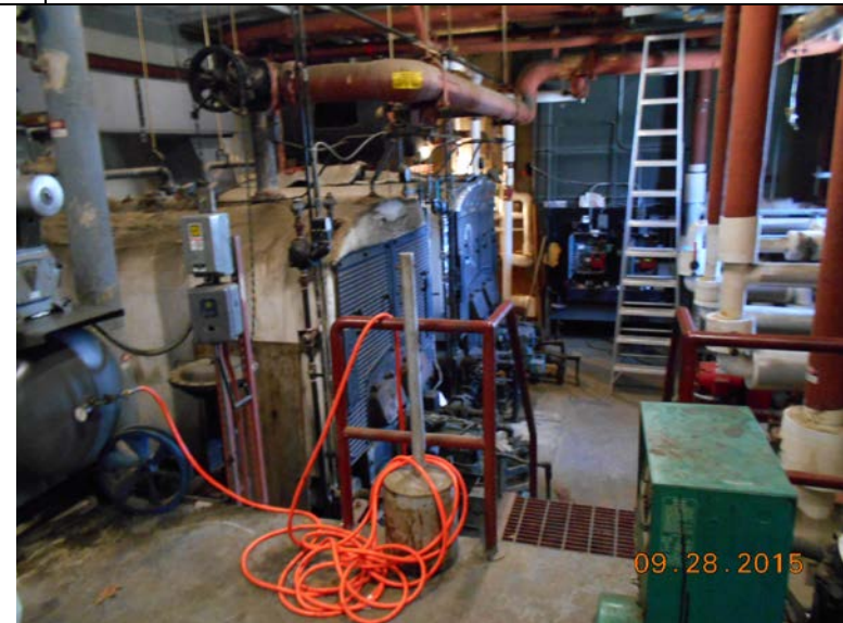
Photo #8: Boiler room
