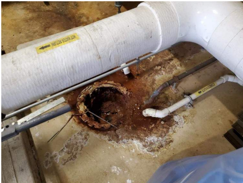
Photograph 30 – Mechanical room drainage with some corrosion.
