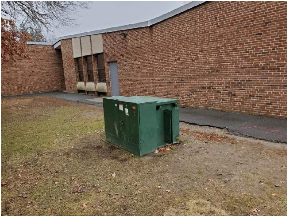
Photograph 33 – Transformer near southwest corner of building.
