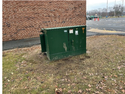
Pad Mounted Transformer
