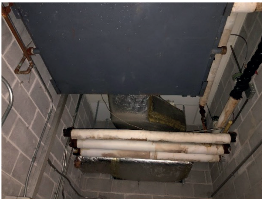
Another original vintage indoor AHU, showing rust perforations along the cooling coil section.
