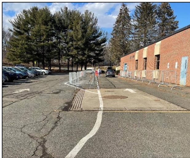
Photo 10: Parent drop-off/pick up loops at the west side of the building. Grade 1-6 parent use the space left of the barricades, kindergarten parents use the right drive aisle and the protected space between the barricades is used as a walkway for Grade 1-6 students.
