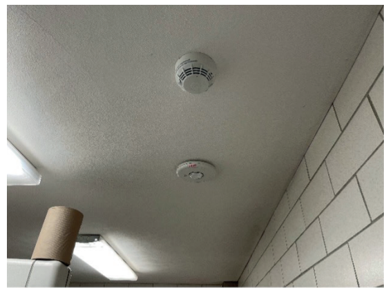
Smoke Detector and Notification Device
