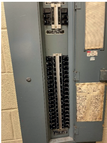
Split Bus Panel
