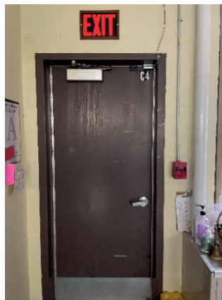
Pull Station at Door
