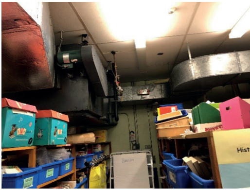
Typical original vintage horizontal indoor Trane air handling unit.
