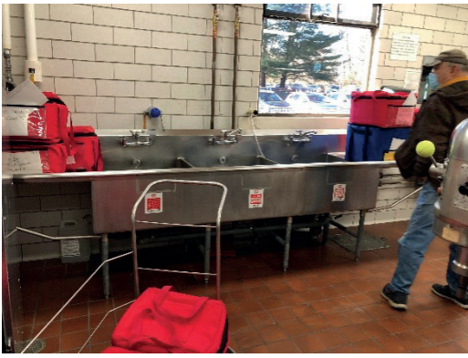
L - Pot sink #1. R - grease trap is underslab and can be serviced.
