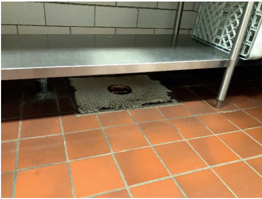
L - Pot sink #2. R - this one also has underslab grease trap but would be pretty difficult to service.
