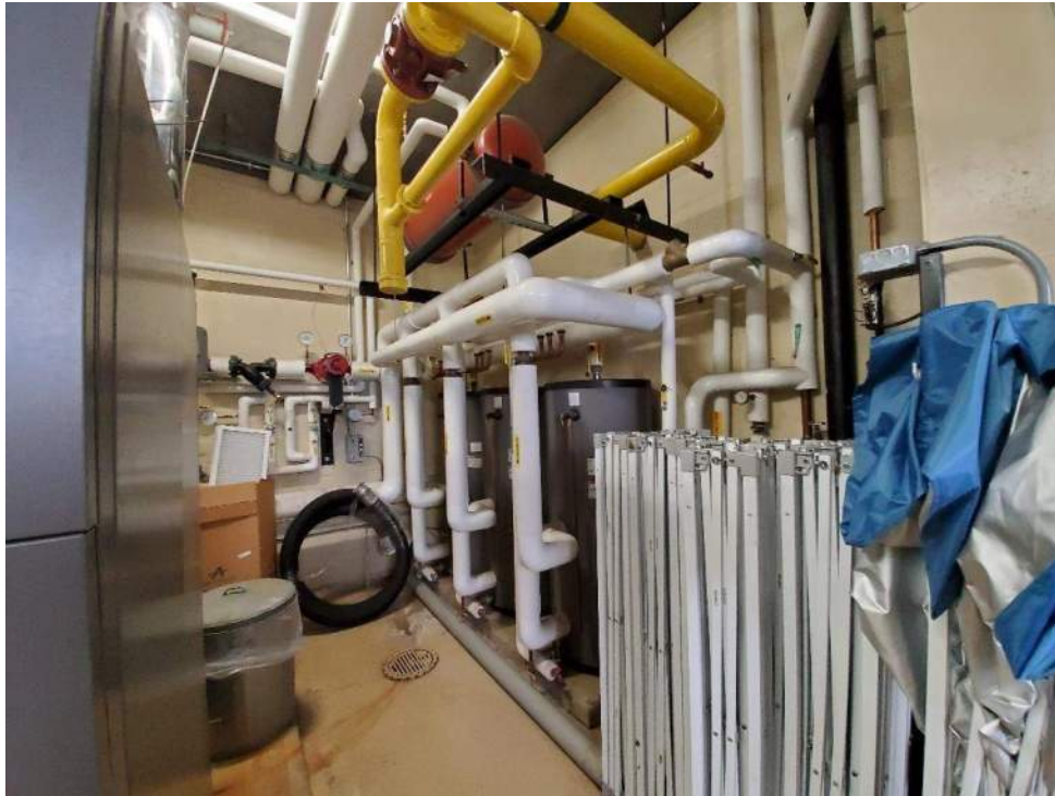
Photograph 31 – Water heaters in mechanical room.
