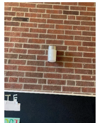
Emergency Only Fixture
