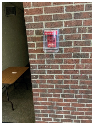
Pull Station not at Door
