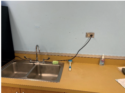
Non GFCI Receptacle at Sink
