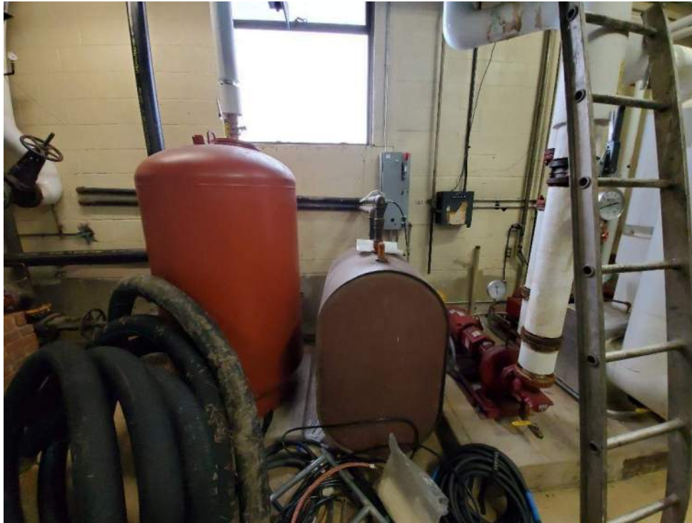
Photograph 29 – 125-gallon diesel tank in mechanical area.
