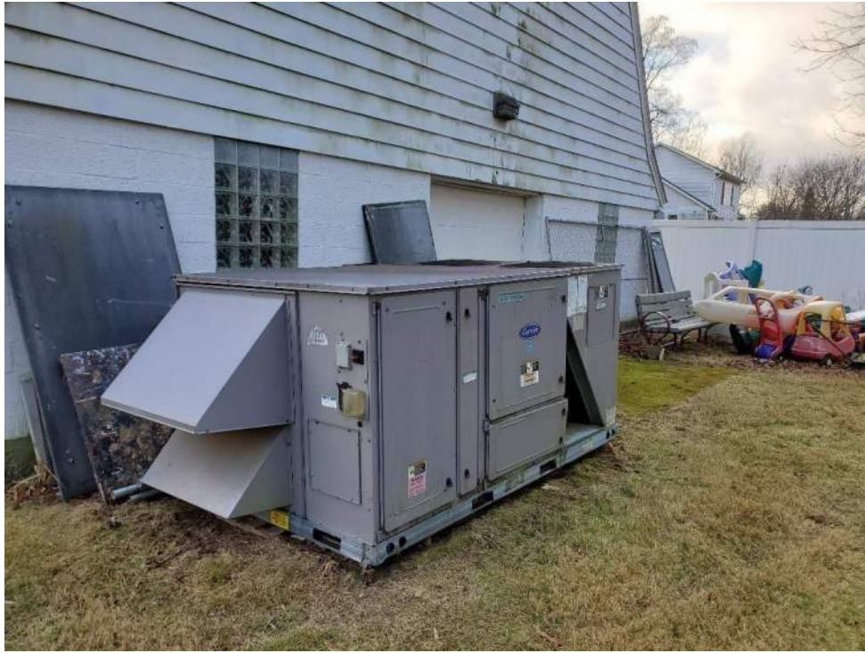
Photograph 35 – Air conditioning unit, no longer in use.
