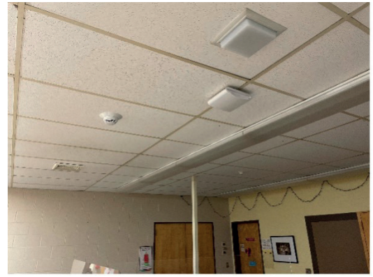
Emergency Only Fixture (foreground)
