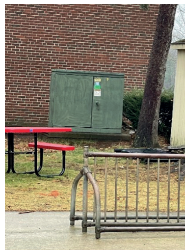
Pad Mounted Transformer
