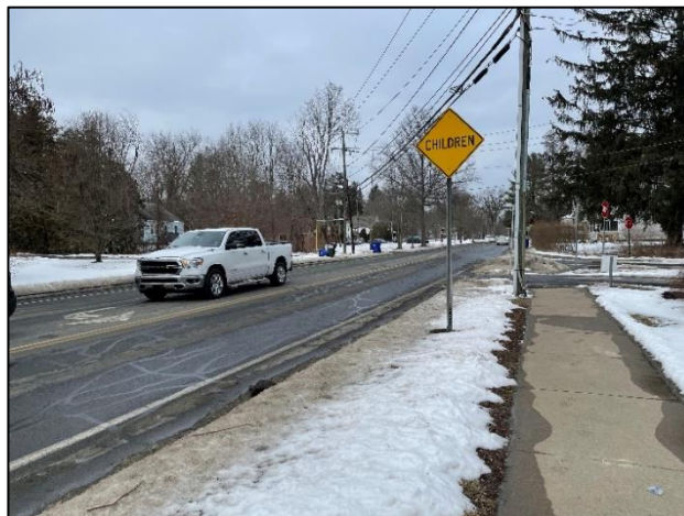
Photo 6: School zone signage along South East Street does not meet MUTCD standards.
