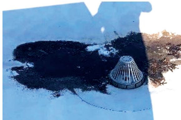
L - roof drain does not have overflow, are connected to internal conductor pipe, and to the under-slab piping to outside the building.
