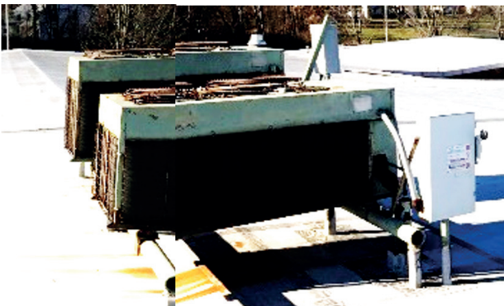
Original vintage air cooled condensing units, which amazingly are still operational, though doubtful reliably or with anyway near the full capacity.
