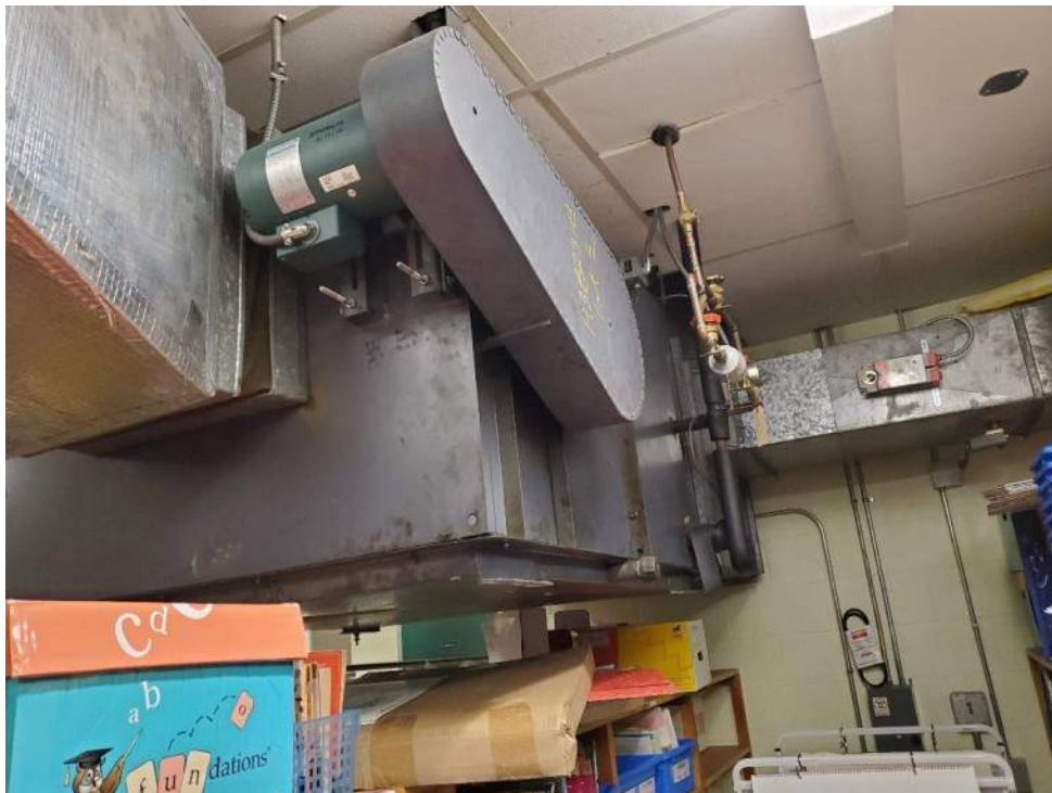
Photograph 24 – Air handling unit in storage closet.
